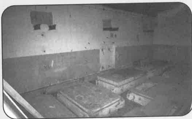
Machinery room for diesel engines and generators
