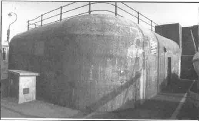
One of the two bunkers along the mole on the way to Castle Cornet (I could have done with an ice-cream). I know they had more time than we did, some four years, but the finish on the concrete is excellent.
