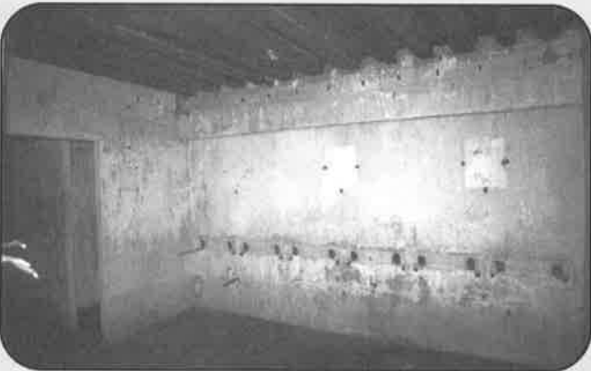
Crew's washroom and toilets, sinks and mirrors gone
