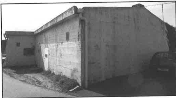
The 319th Communications H.Q. bunker, just over the road from the other two in a street named Les Quatre Vents. It now makes an excellent thief proof store !
