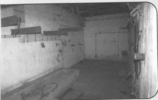
Air conditioning compressors and fridge unit room
